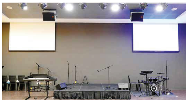
The Agape Hall has been upgraded with a Norton coaxial speaker system
