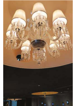
Eiki EK-401W video projectors have been installed into each of the eight chandelier recesses
