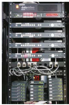
VGA, HDMI and audio outputs from seven wall plates are scaled before being processed in the Kramer VS-88HDx1 matrix
