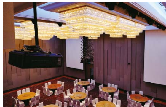
40 Martin MH1 Profile moving heads have been programmed using Crestron software
