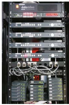
VGA, HDMI and audio outputs from seven wall plates are scaled before being processed in the Kramer VS-88HDxl matrix
