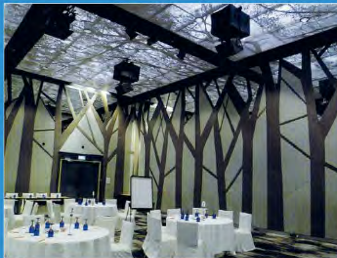
The ballroom now benefits from two ceiling suspended I12 enclosures with I118B subwoofers
