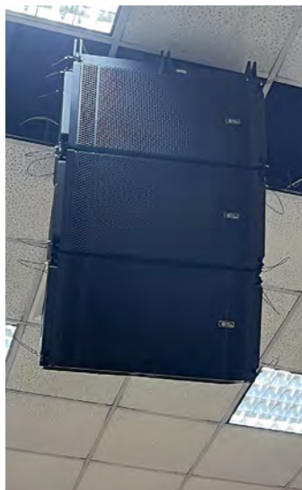
The main line array consists of three Alpha Acoustics KROSS 7 speakers each side
