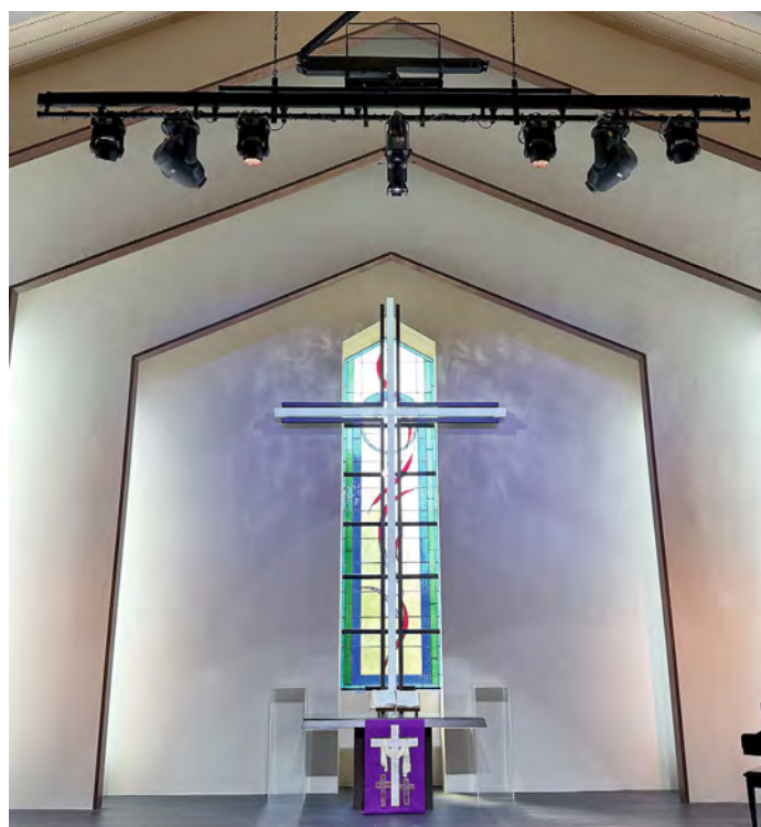
Martin LED moving heads assembled on two overhead bars
