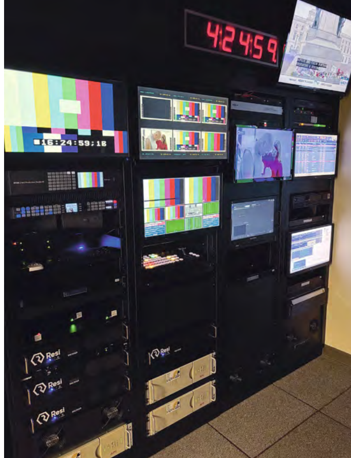
GABC's TV master control as it looks today
