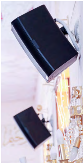
Just short of 100 QSC speakers have been installed at Burhani Masjid
